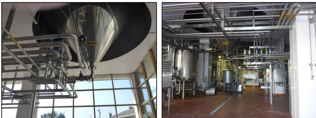
Plates 63-64 Maturation Building internal workings
